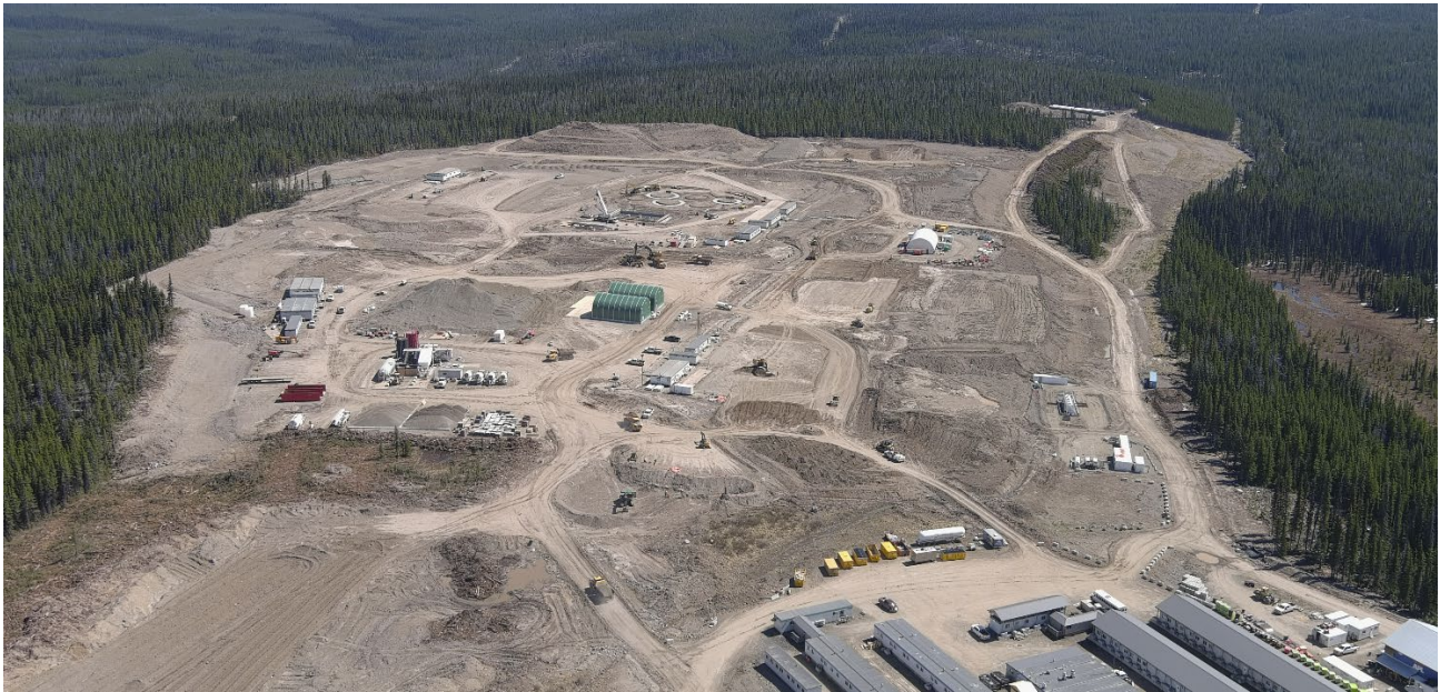
Processing Plant Area at Blackwater Mine – May 2023
