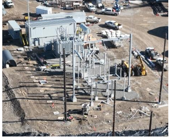
25kV electrical substation and 225kV transformer
